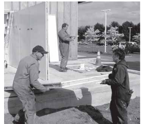
BCS maintenance employees, Bob Hickok (Left) and Brad Klein, tilt up another freezer wall in the foreground while Chuck Osborn carefully loads the next cartridge of caulking.
