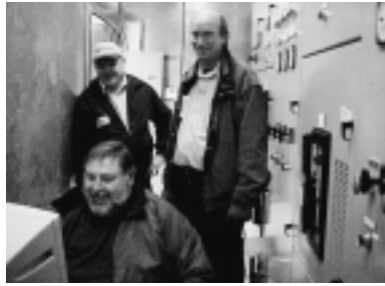
Mike Clausen working inside the natural gas units with Simpover employees Gordon Carlton and Kerry McDonald looking on with support.
